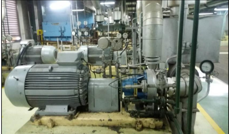
Gambar 3.1 Low Pressure Boiler Feed Pump PLTGU Blok I PT. PJB UP Gresik
