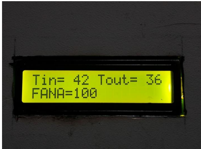
Gambar 4.5 Display LCD kondisi Fan Cooling Tower 100%
