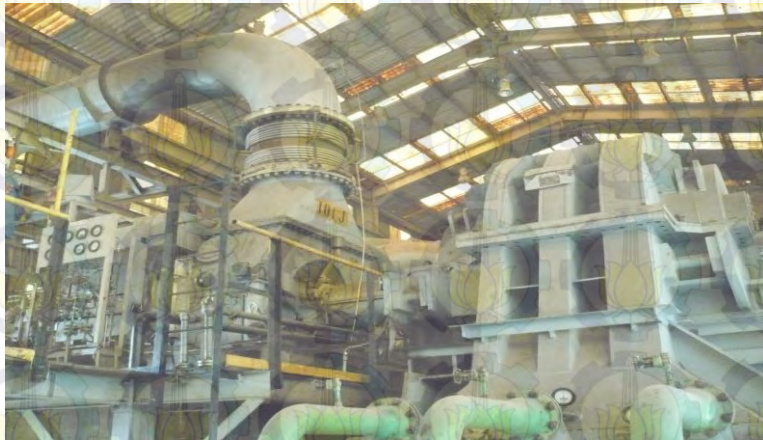
Gambar 2.7 Air Compressor 101 J
