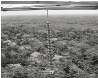
Gambar 3.5 Insulator tipe I String
