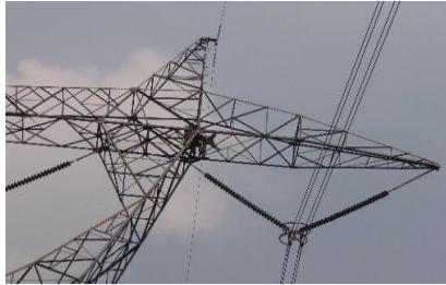
Gambar 3.6 Insulator tipe V String
