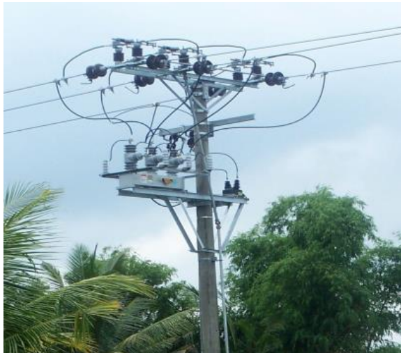
Gambar 2.2 Recloser di lingkungan kerja UP2D
