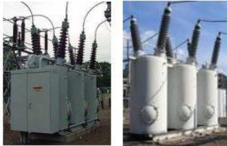
Gambar 2.1 Oil Circuit Breaker
