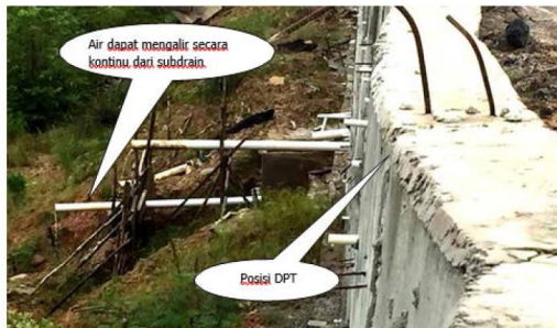
Gambar 1. 8 Kondisi subdrain (Sumber : GEC 2018, Report ReviewGrand blpp)
