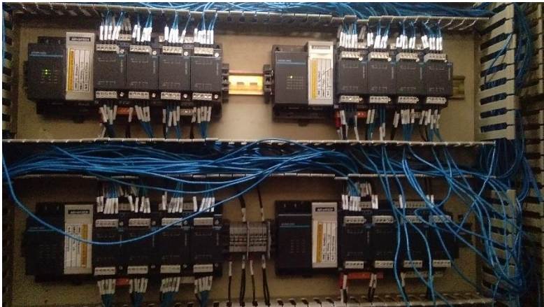
Gambar 2.2 RTU I/O Advantech
