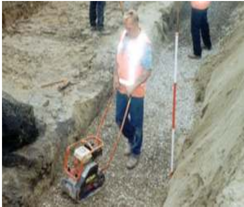
Gambar 5.10 Perbaikan tanah dasar Segmental Blok Sumber : Commercial Installation Manual for Allan Block Retaining Wall
