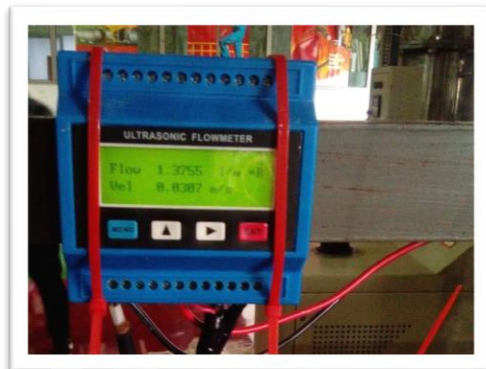
Gambar 10. Tampilan Ultrasonic Flowmeter TUF-2000M
