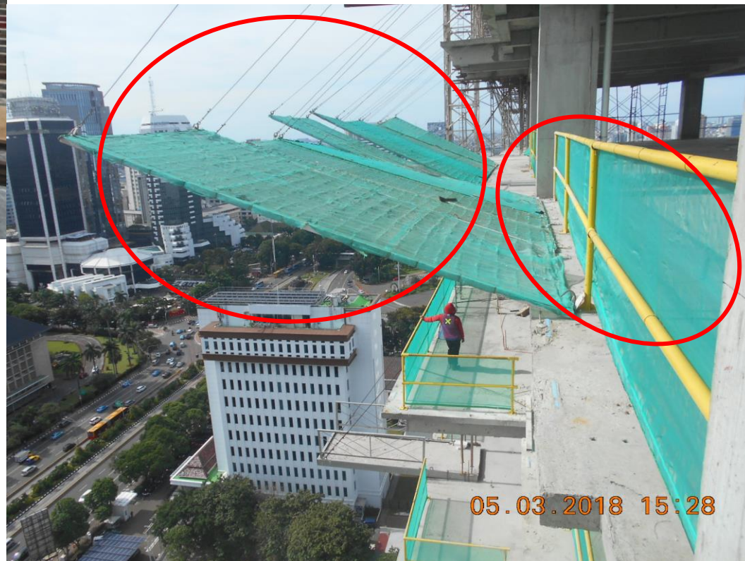
SAFETY DECK DAN RAILLING
