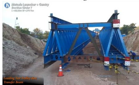
Sumber: PT. Jatra Sejahtera Gambar 4. 40 Loading Test Trolly dan Transferred Beam/Rel Geser
