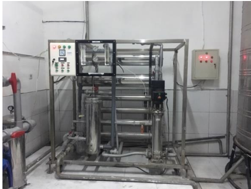
Gambar 4.3 Unit Reverse Osmosis
