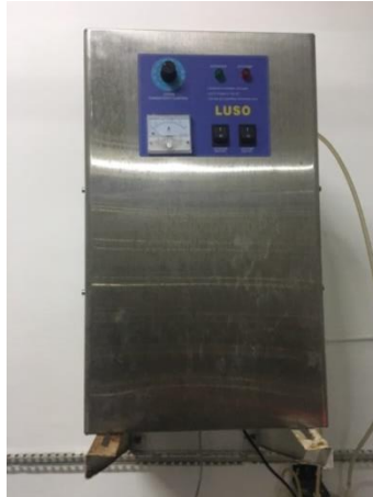
Gambar 4.4 Unit Ozone Generator
