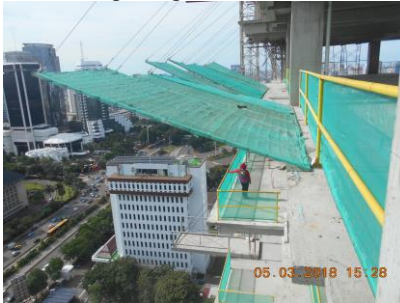
Gambar 5. 10. Pagar Pembatas ( Guard Railing ) [11]
