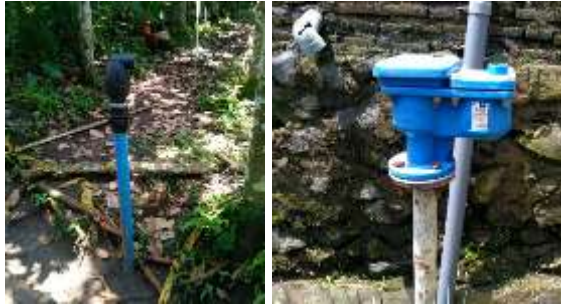
Gambar 4.6 Air Valve Eksisting
