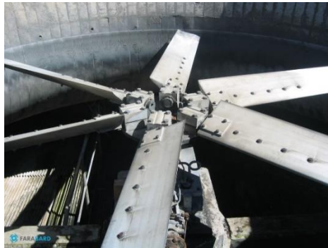
Gambar 2.6 Fan pada Air Cooled Heat Exchanger (Farabard.IR, 2019)
