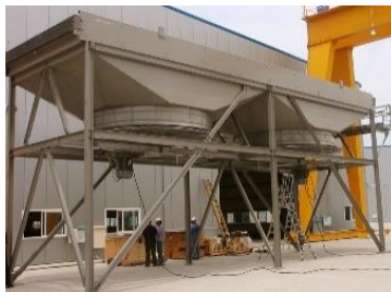
Gambar 2.3 Air Cooled Heat Exchanger (Technologies, 2019).
