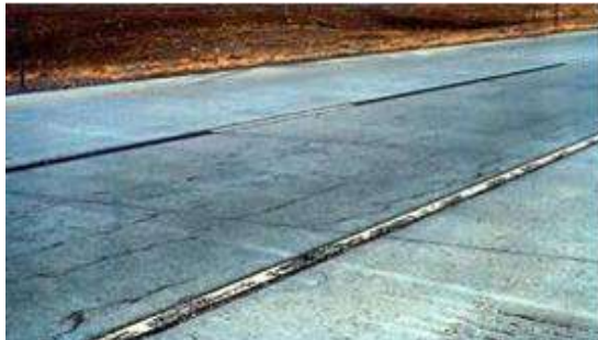
Gambar 2.8 Retak susut ( shrinkage crack ) Sumber : Ziantono, 2016
