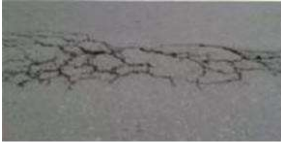
Gambar 2.1 Retak Halus (hair cracking)
