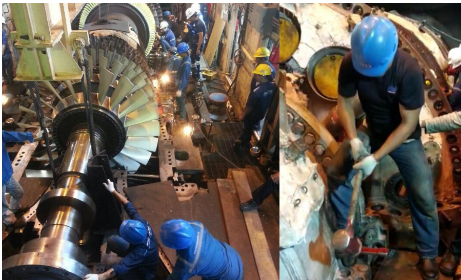
Gambar 2.4 Ilustrasi pelaksanaan overhaul Major inspection Gas Turbine
