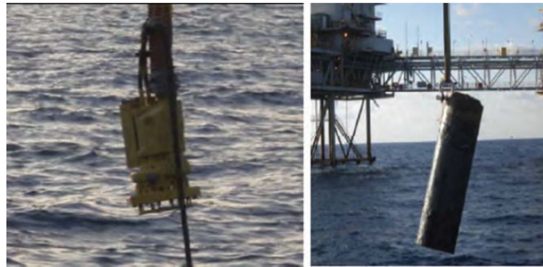
Gambar 2. 9. Member Removal pada Subsea Casing Stub di Gulf of Mexico (Sumber: Nichols dan Khan, 2017)
