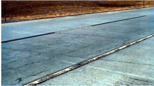
Gambar 2.8 Retak susut ( shrinkage cracks )
