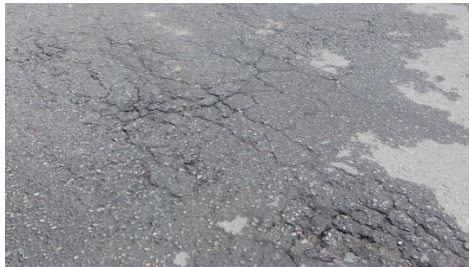
Gambar 2.1 Retak halus ( hair cracking )
