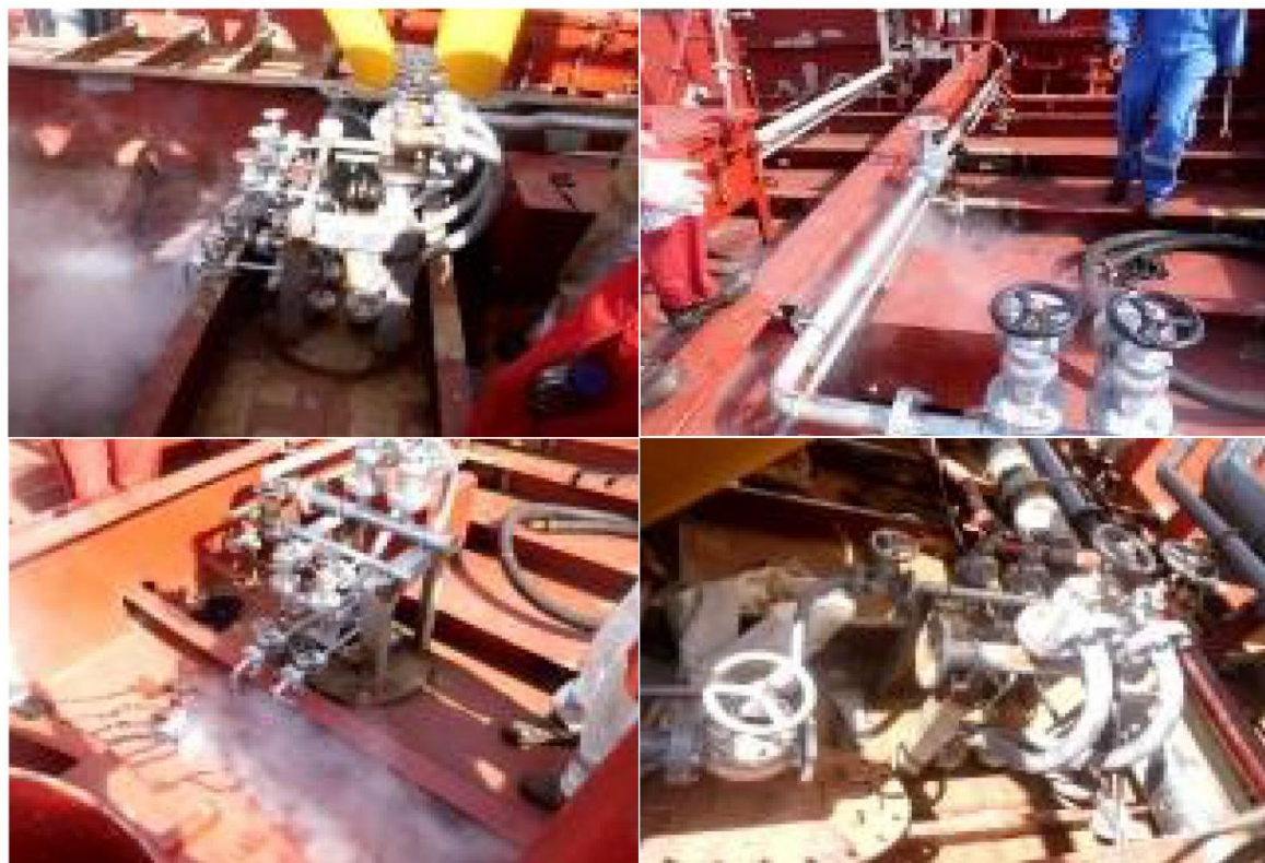
Gambar F.1 Heating Pump Commissioning
