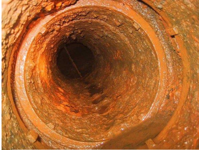
Gambar 2. 5 Internal Korosi pada Pipeline (Sumber : https://www.pipingengineer.org )
