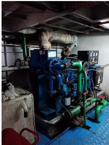
Gambar 3.3 Ruang Generator Natuna Express
