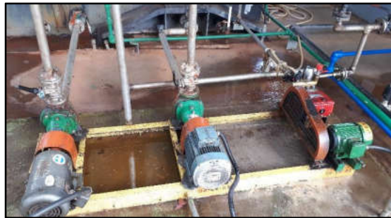
Gambar 4.1 Pompa Scrubber, Quencher dan Waste
