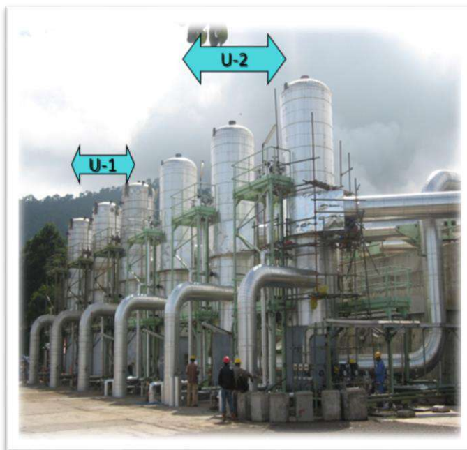
Gambar 2. 7. Separator Station di PLTP SEGWWL
