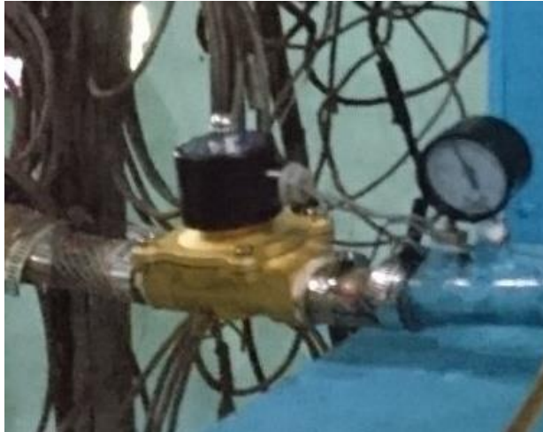
Figure 3.4 Solenoid Valve for temperature control
