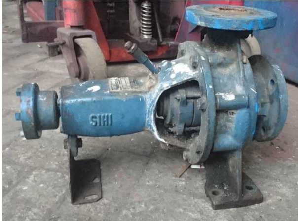
Figure 3.9 Water Brake cooling pump needs a bearing change
