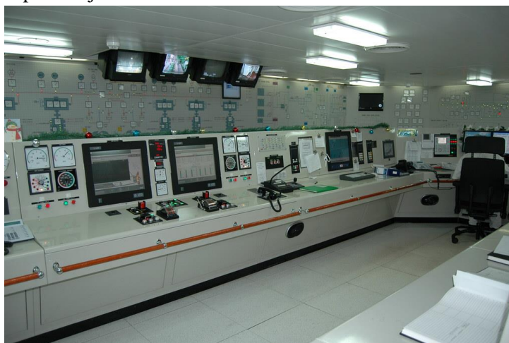
Gambar 2. 1 Engine Control Room
