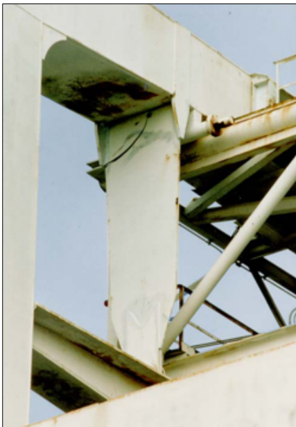
Gambar 4. 5 Crack akibat fatigue (Sumber: www.liftech.net )
