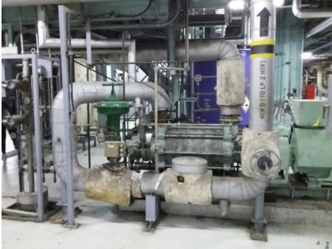
Gambar 2 Heater Drain Pump ( Heater Drain Pump PLTU Unit 3 PT PJB UP Gresik )
