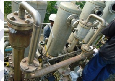
Gambar 4.12. Pengecekan Vacuum Unit
