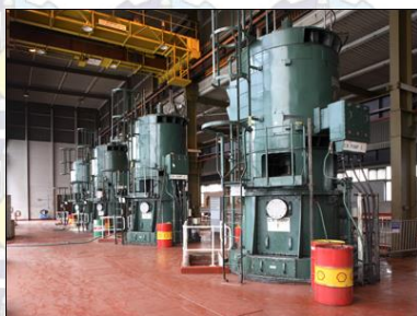
Gambar 2.4. Circulating Water Pump
