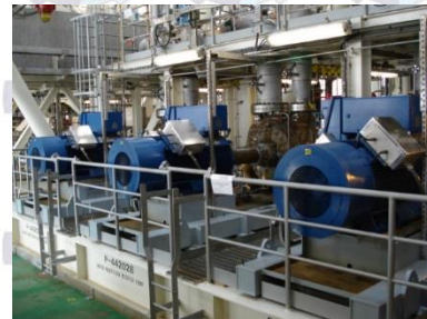
Gambar 2.5. Sea water Booster Pump
