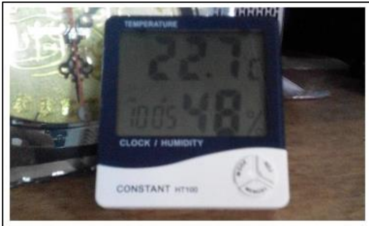
Gambar B.38 Sensor Suhu Ruang Server
