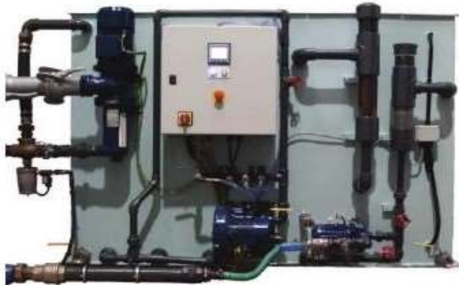
Gambar 5. 37 Sewage Treatment Unit FBBR 50
