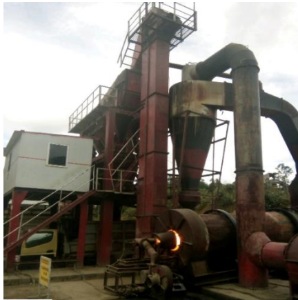
Gambar 2. 15 Asphalt Mixing Plant
