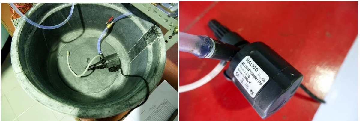
Pompa, Valve, dan Reservoir
