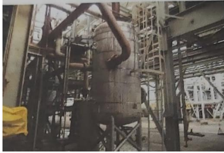
Figure 2.2 Blow Off Tank
