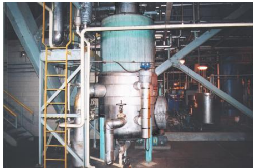
Figure 2.1. Continuous blowdown tank Source:magnetrol.com
