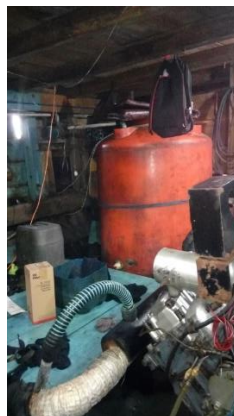
Figure 4.3. KM Izhar Engine Room
