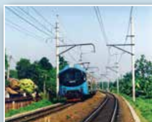
Railway Catenary Poles
