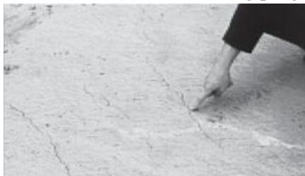
Gambar 2.4 Plastic shrinkage cracks (National Ready Mixed Concrete Association)
