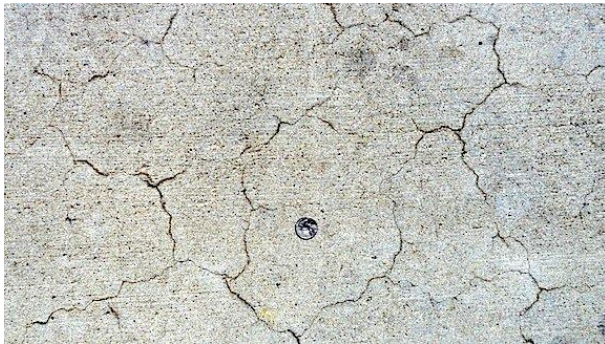
Gambar 2.6 Crazing concrete surface (Sumber: google.com)
