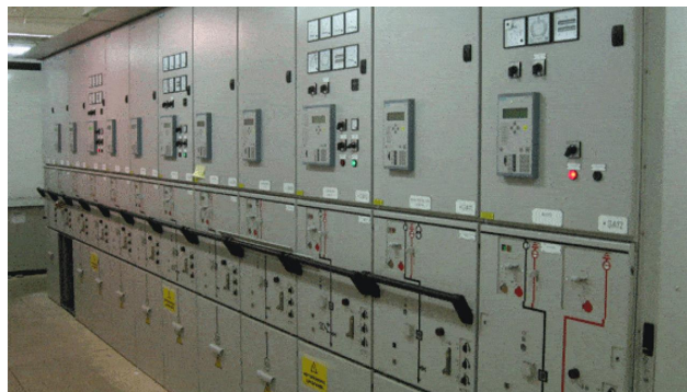
Gambar 2.20 Main Switch Board
