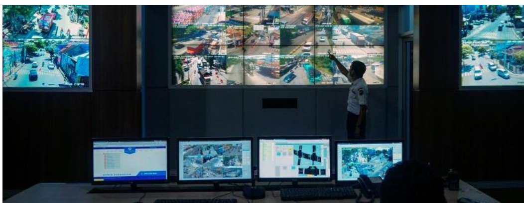
Gambar 2.5 Ruang Area Traffic Control System (ATCS)
