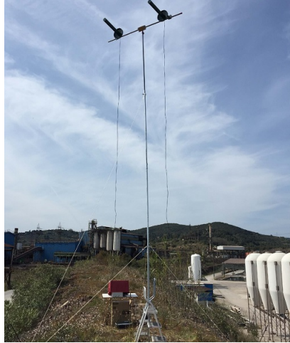
Gambar 2.17: Gateway menggunakan Antenna Digital Outdoor di Laut Tyrrhenian, Italia [13]
