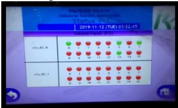
Gambar 4. 4 Status PLC P3 Infeed Panel
