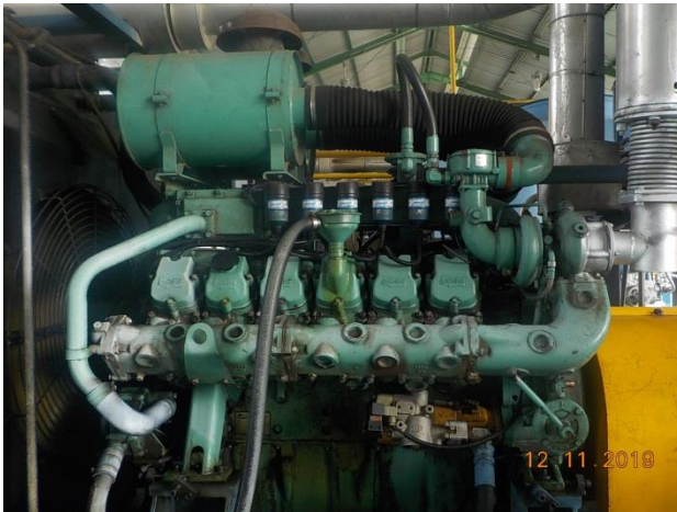
Gambar 2.2 Gas Engine Tipe GV222TIC (PT PERTA DAYA GAS)
