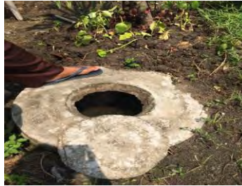
Gambar 5.18 Sumur Resapan Puskesmas Tanah Kalikedinding
