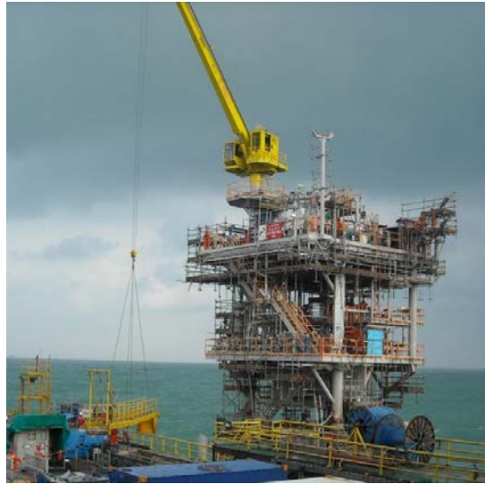
Gambar 3.4. Wellhead Platform UL A PHE ONWJ (PT. BKI (Persero))
