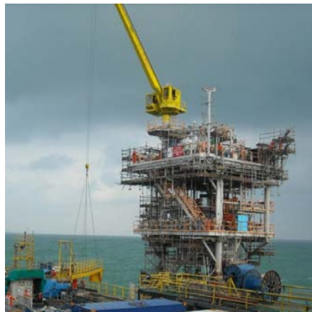
Gambar 1.3. Wellhead Platform UL A PHE ONWJ (PT. BKI (Persero))
