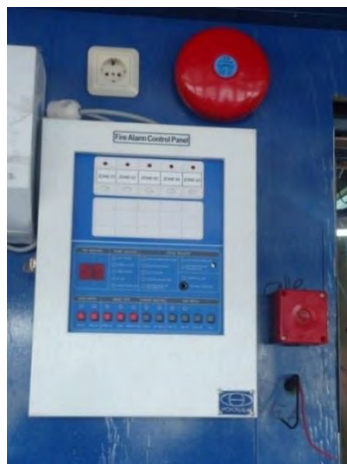
Gambar II. 11 Fire alarm panel
