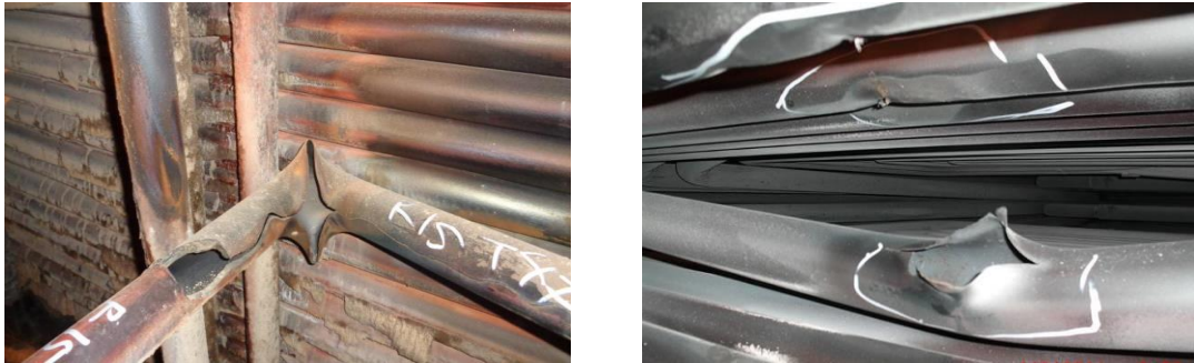
Gambar 2.8: Kerusakan tube akibat overheat
