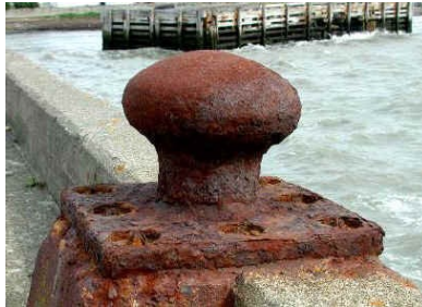
Gambar 2.2. Korosi uniform (API 571)
