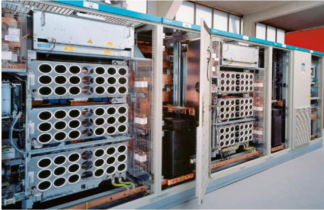
Figure 0-2 SIPLINK with open cabinet doors
