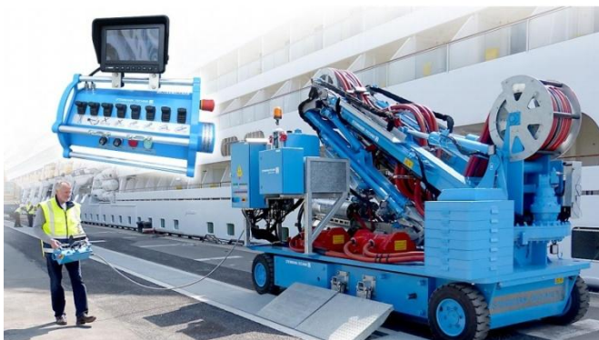
Figure 0-11 Control panel to move the robot arm into ship's power plug
