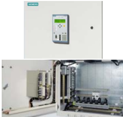
Figure 0-10 Low voltage compartment
