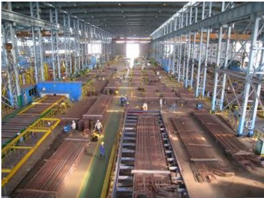
Gambar 4.1. Proyek Coal Fired Boiler.(koleksi pribadi)
